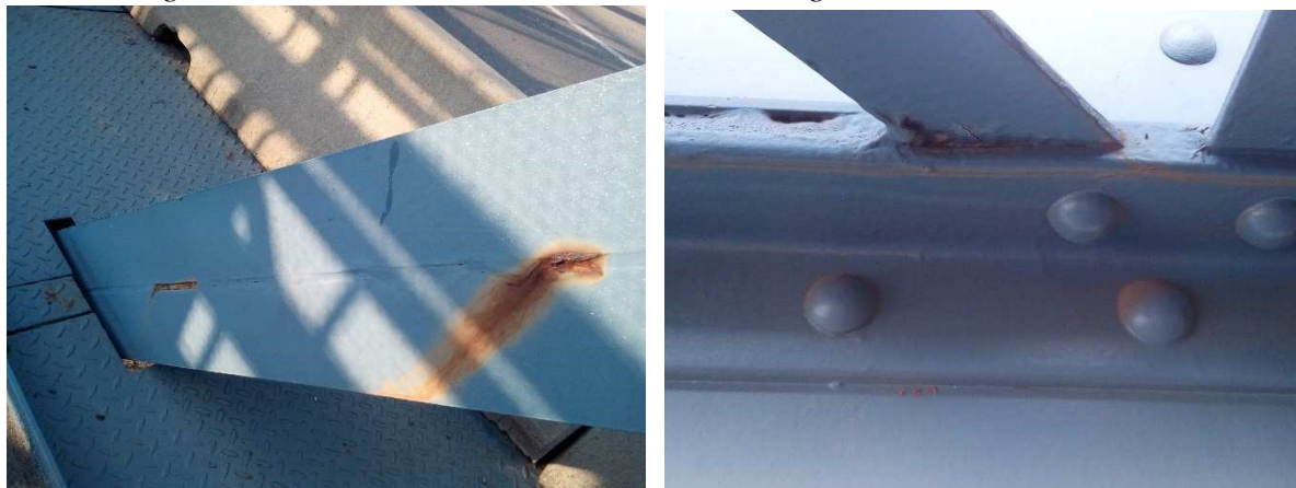
Fig. 5: Defects 13 years after reconstruction (photo from 2018) [SUDOP photo] 2.2.2 Railway viaduct Chrást (Plzeň-sever) [11]
