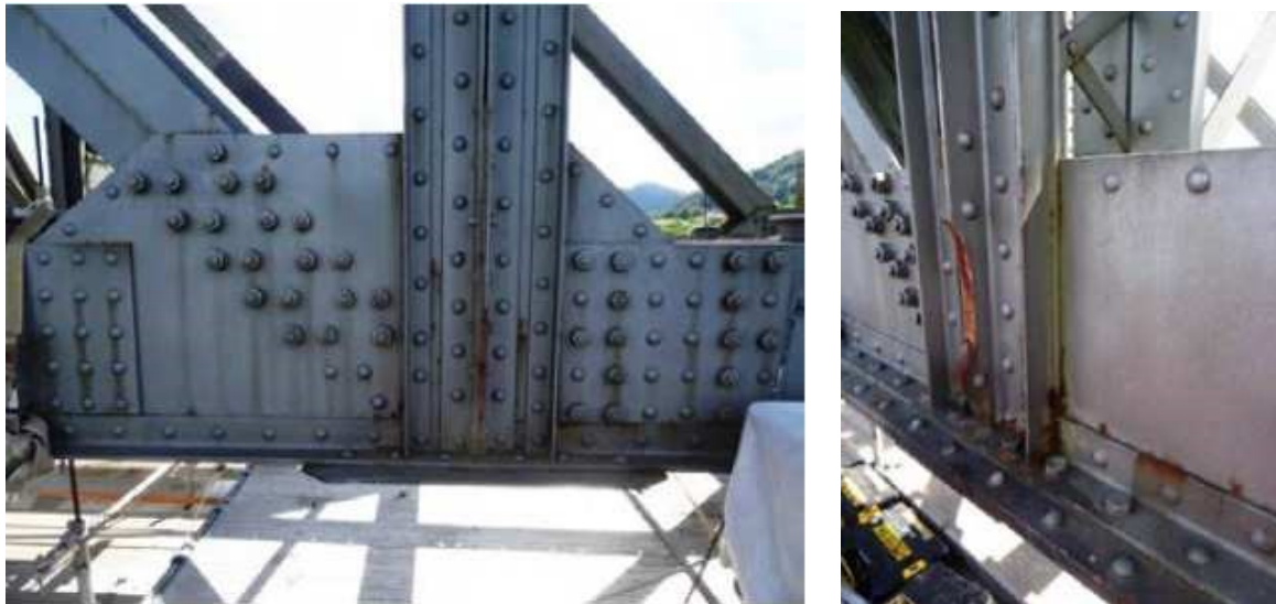
Fig. 24: View of the structure before the blasting – CPC on the surfaces is still functional, local corrosion is occurring, corrosion losses are still negligible
