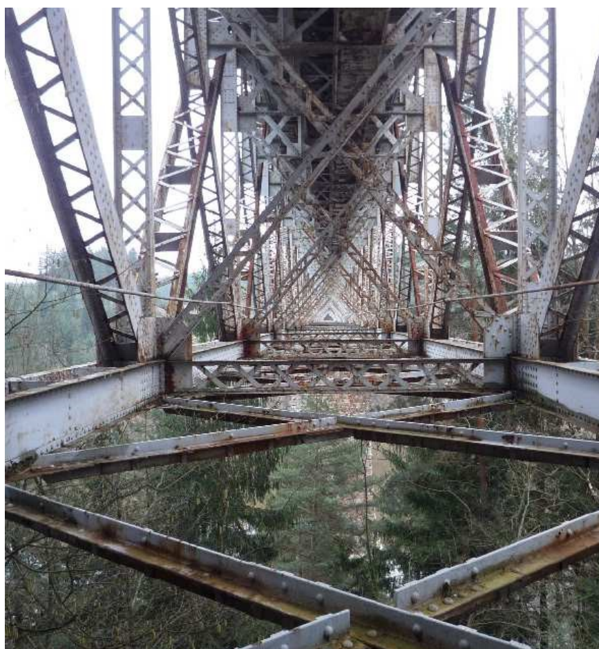
Fig. 11: View of the bridge axis at the level of the lower chord
