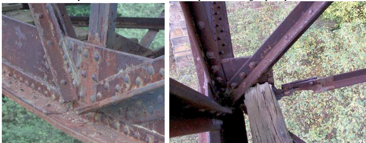
Fig. 8: Details of the bridge structure before repair
