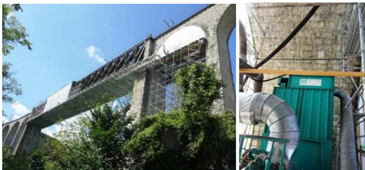
Fig. 23: Airtight canvas covering, right view inside the canvas covering
