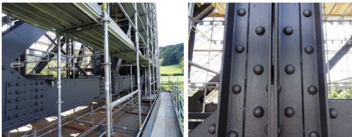
Fig. 25: View of the structure after application of the new CPC, on the right it is shown that it is possible to clean and apply CPC even in the narrow space between the plates without filling the joint
