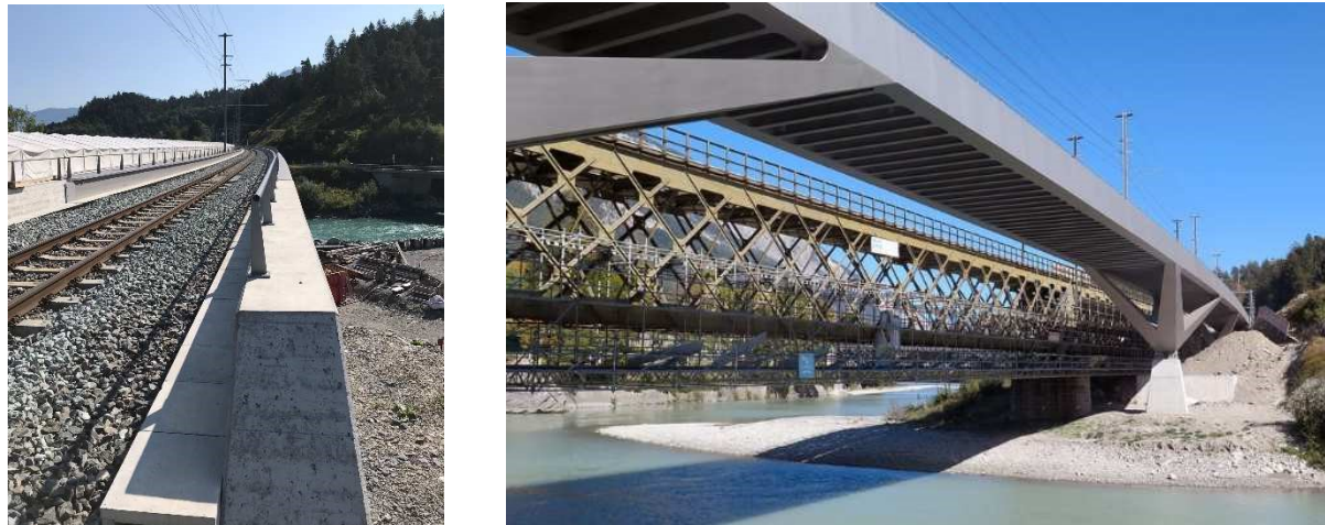
Fig. 31: Pictures showing an example of a implemented single-track steel bridge Zweite Hinterrheinbrücke in Switzerland near Chur (Load-bearing structure of 2 steel beams 1.7 m high, 0.5 m above the rail grade line, trough for railway bed, diagonal braces, span of bays approx. 46.5 – 40.1 – 63.0 – 45.9 m)
