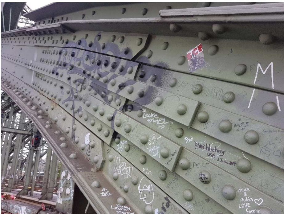
Fig. 20: Detail of the arch area with a high concentration of riveted joints and scabs
