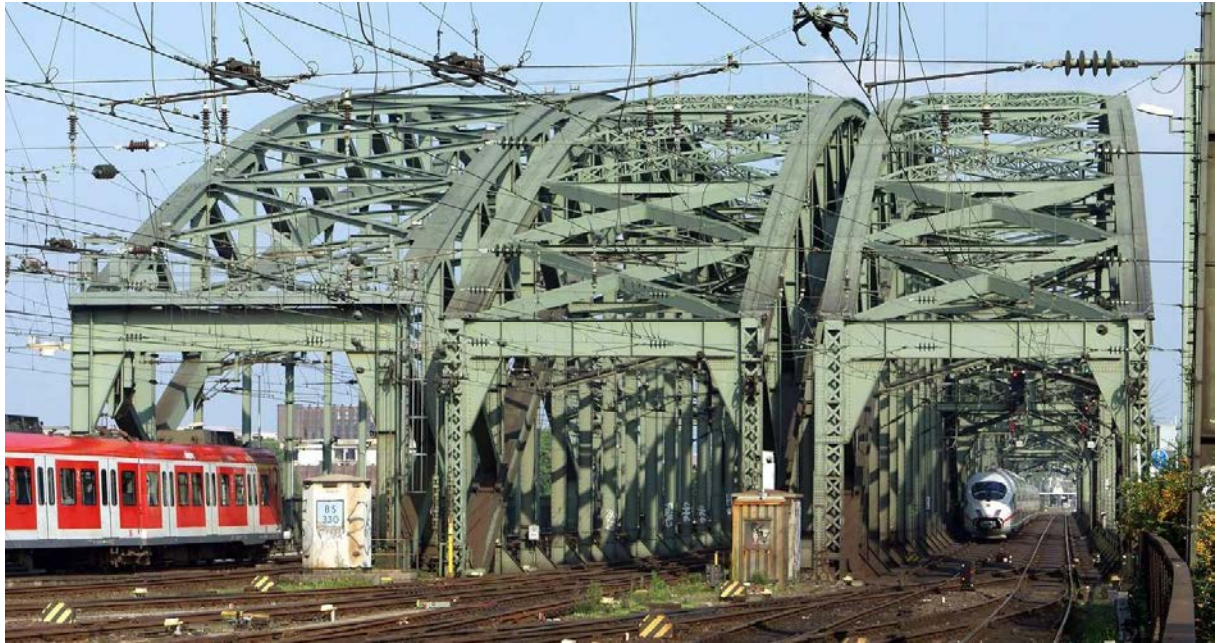
Fig. 17: Different structural designs of each of the three double-track bridges evident from the differences in the extreme portal frames
