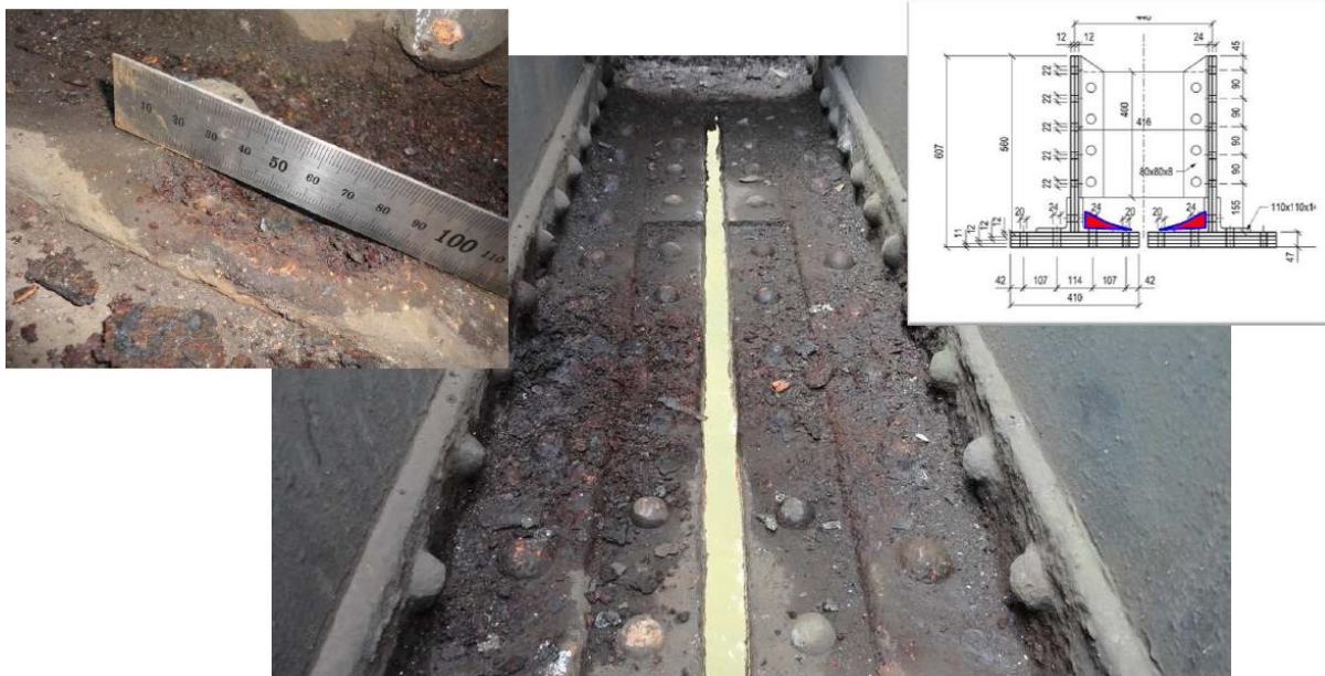
Typical corrosion of the lower chords of the main beam
