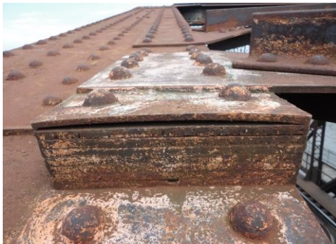
- DEFORMATION OF THE SPLICE PLATE STIFFENING CONNECTION
