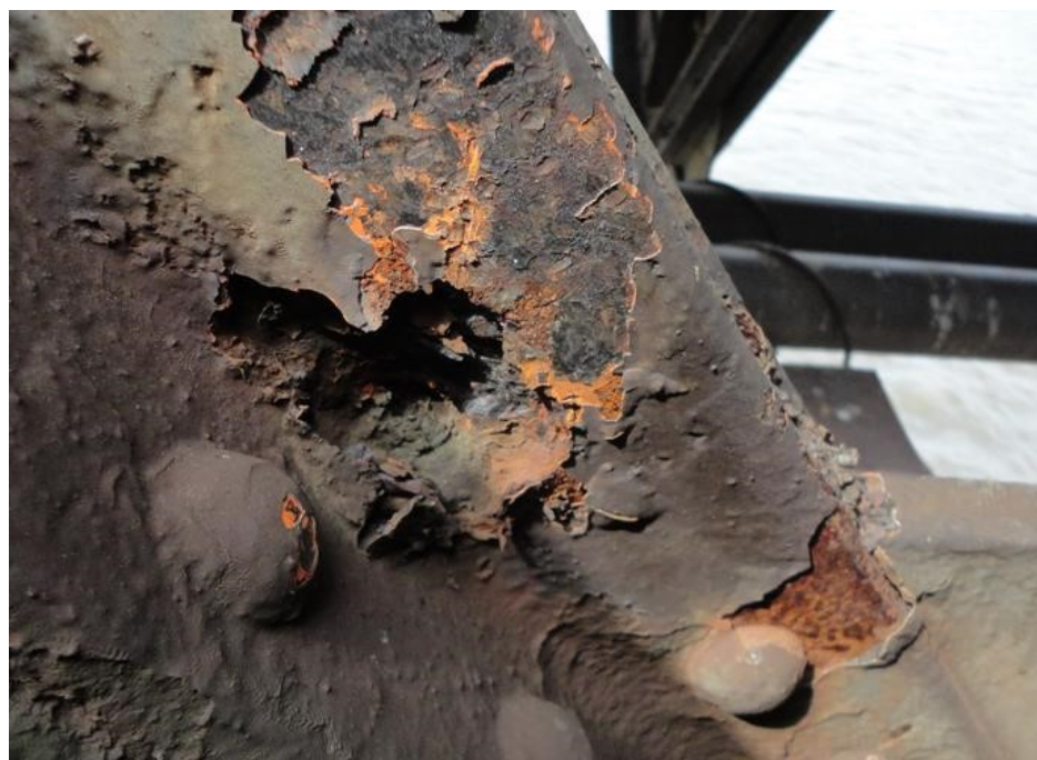
Corrosion at the connection of the lacing (NK2 – right D.7) to the splice plate of the lower chord U.7
