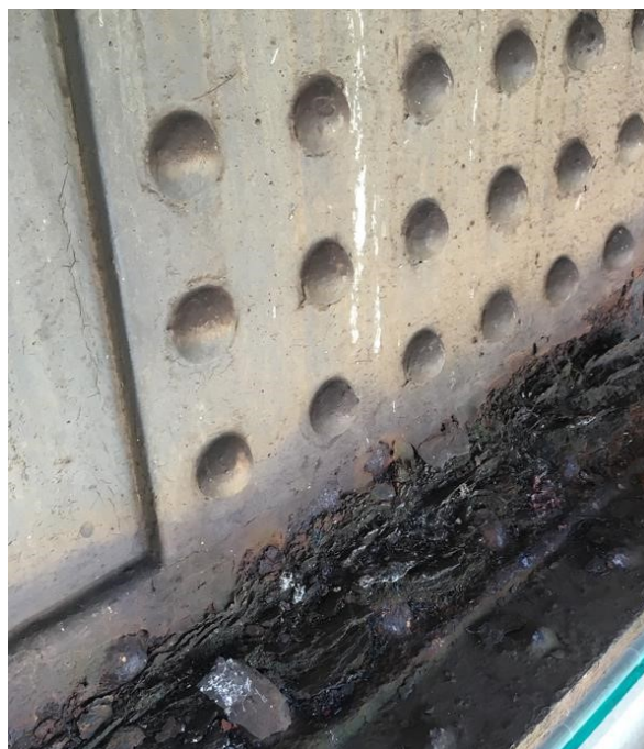
Corrosion of the neck angles of the lower chords in areas with constant moisture
