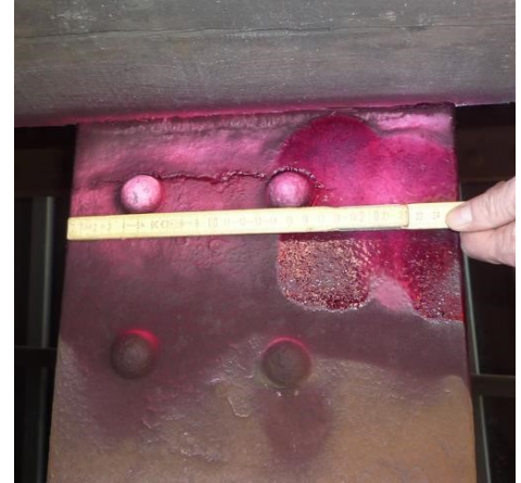
crack in the longitudinal truss chord L4.1 (NK1)
