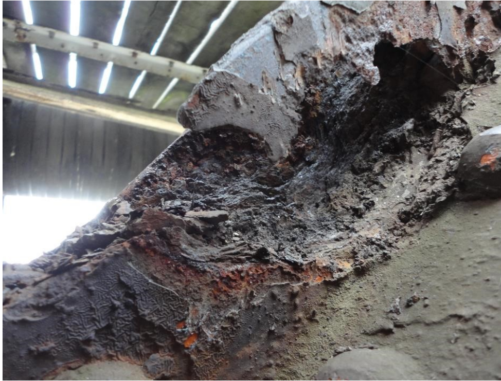
Corrosion at the connection of the lacing (NK1 – right D.7) to the splice plate of the lower chord U.7
